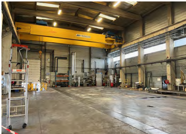
Disassembly of the 5400-tonne press in order to accommodate a new, more efficient press.
