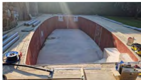
Renovation of a 1980s swimming pool – 9x4m traditional filtration with sprayed-polyester panels.
