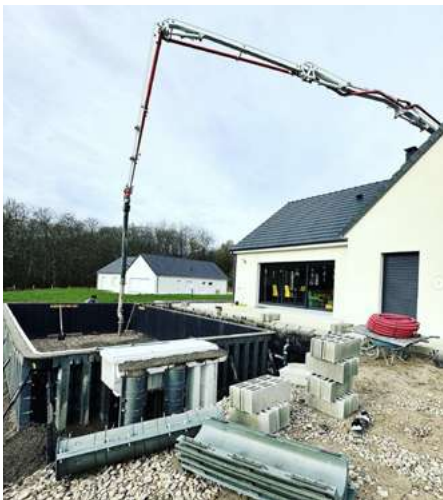
Casting underway for a creation by Teillais Piscines by Mr Teillais in Plaimpieds-Givaudins (Cher).
