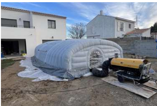
Piscines Sud Evasion in Salon-de-Provence (Bouches-du-Rhône) was able to place this liner in the middle of winter thanks to a construction-site shelter.
